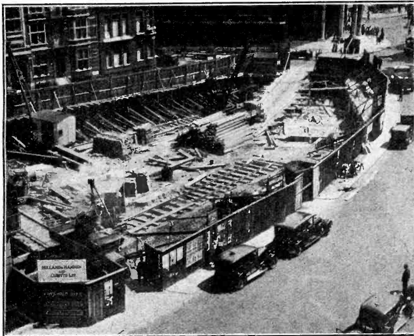
FUTURE HOME OF BROADCASTING. Work has now begun on the erection of Broadcasting House, Portland Place, London, W. The photograph shows the preliminary excavations in progress. Part of the Queen's Hall can be seen in the background on the right.
